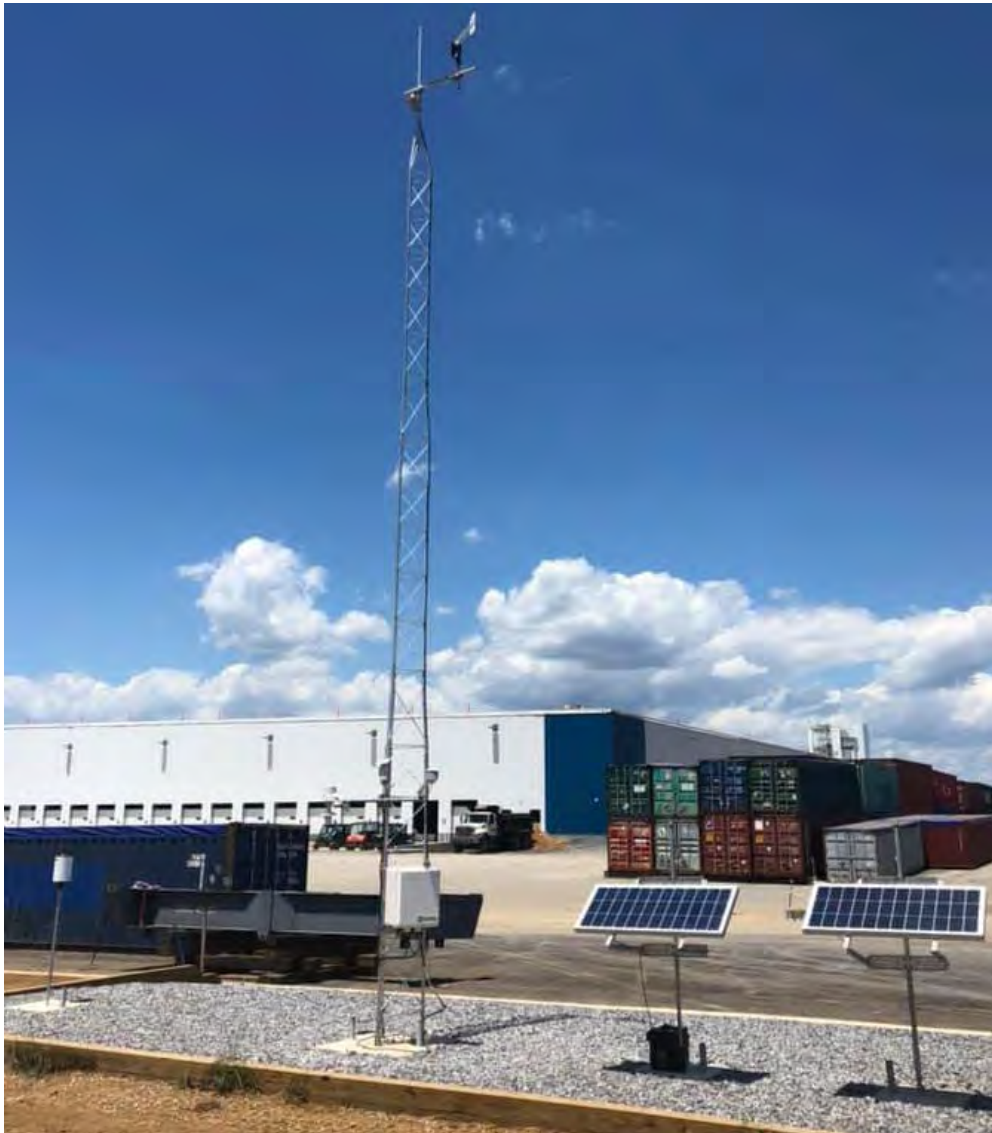
Figure 4: ROCKWOOL Meteorological Monitoring Location
